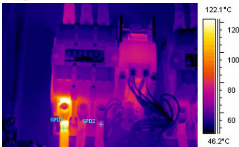
Figure 17.9 An infrared image of indoor electrical equipment (2).
