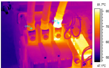
Figure 17.8 An infrared image of indoor electrical equipment (1).
